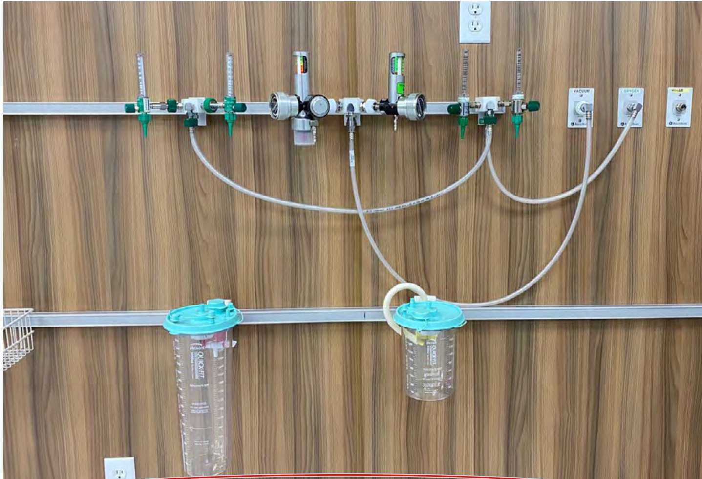
Figure 2-11: Medical Gas Expansion Rail
