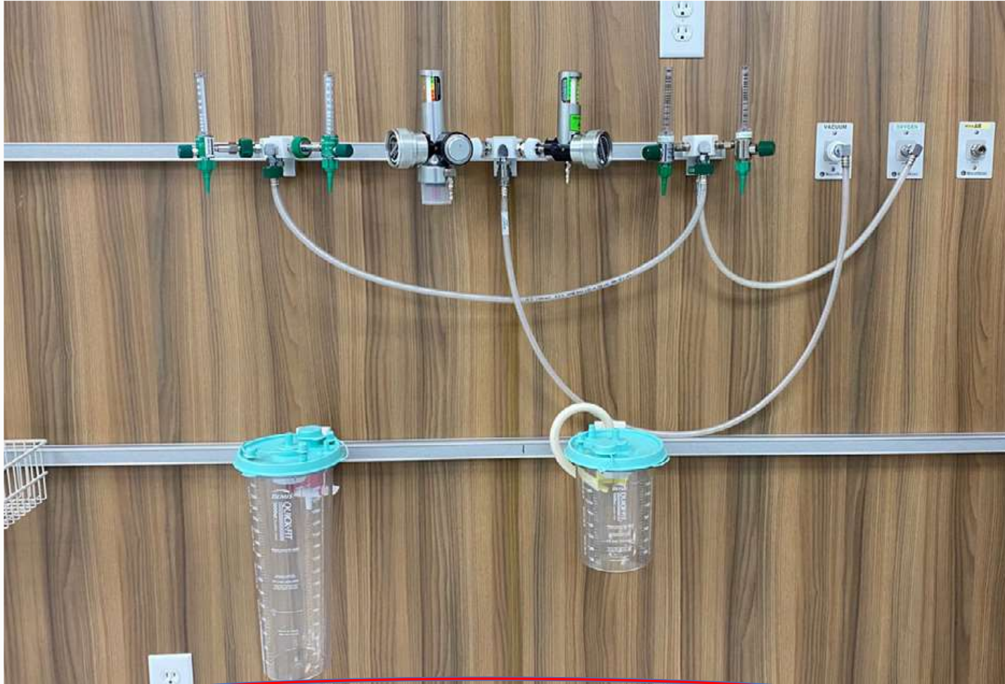
Figure 2-11: Medical Gas Expansion Rail
